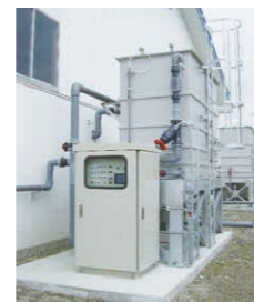
Water purification systems
