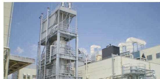
Solvent recovery system (product of Kureha Engineering Co)
